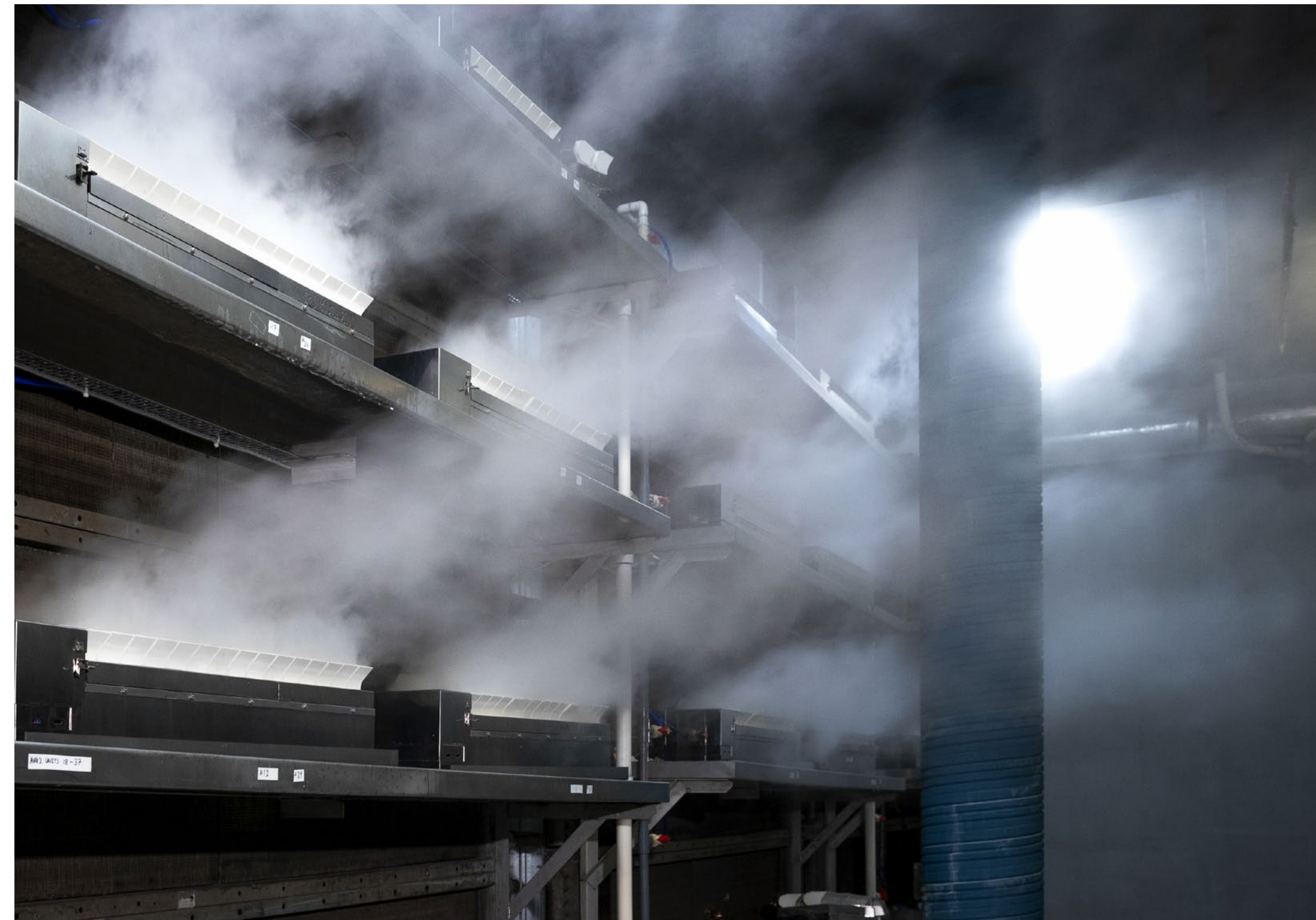
The installation of an ultrasonic humidifier to the Air Handling Units in 2019 has improved energy efficiency and system performance.
